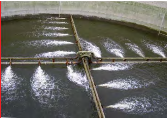
JET MIXING IN EQUALIZATION TANKS
