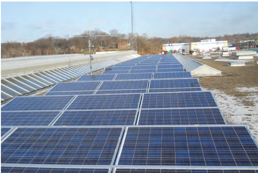
Solar panels installed on the roof of Greater Cincinnati Water Works
