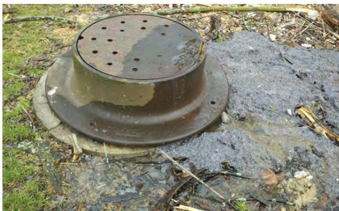
Sanitary sewer manhole overflow
