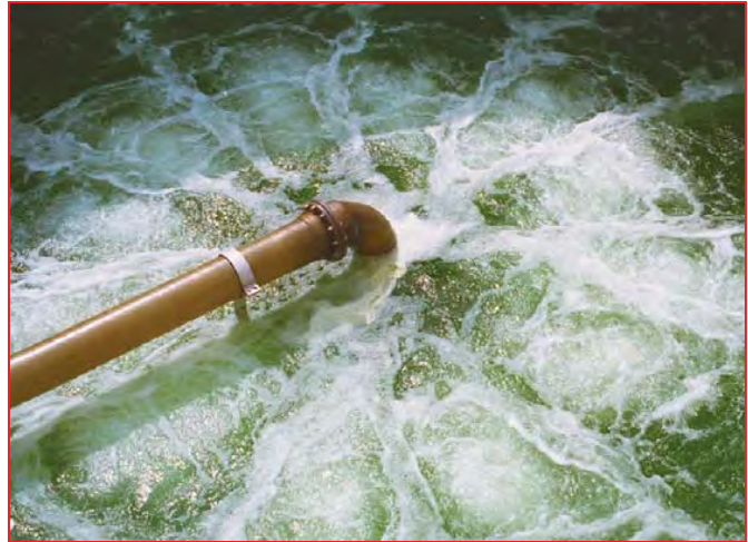
MIXING AND AERATION IN pH CONTROL TANK
