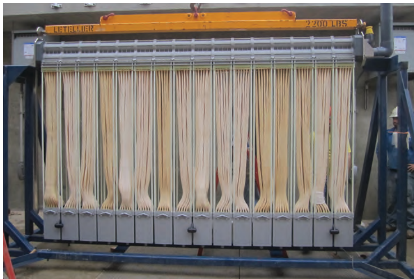
Membrane filter rack
