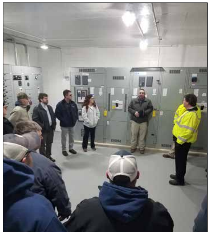
Tour of the newly upgraded Village of Commercial Point WWTP during February Section Meeting.
