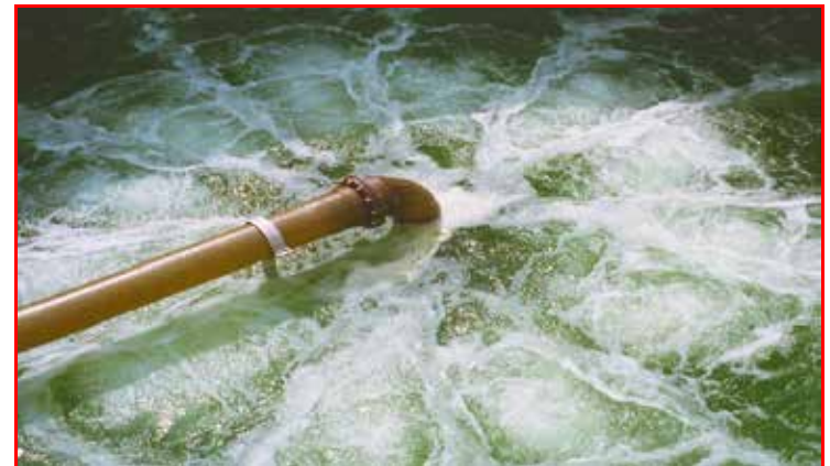
MIXING AND AERATION IN pH CONTROL TANK
