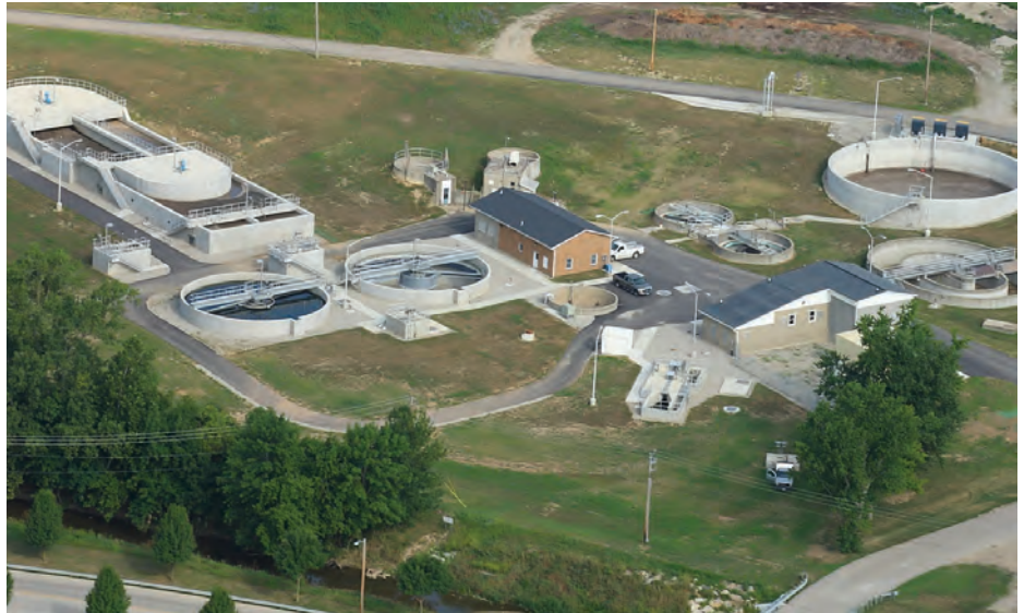
Figure 1: Versailles, OH Water Reclamation Facility
