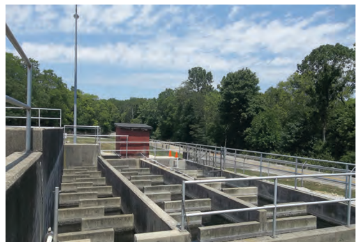
Chlorine contact tank
