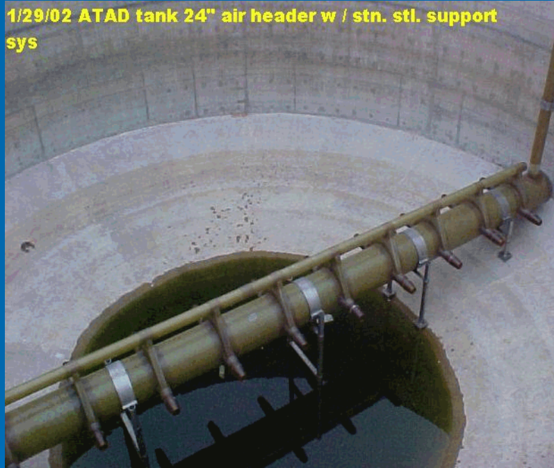
4/19/02 ATAD/ 24" air jet manifold in action at ATAD tank
