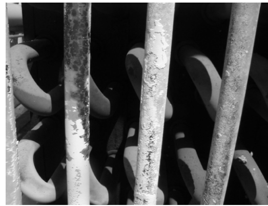
Siloxane deposits on tubes
