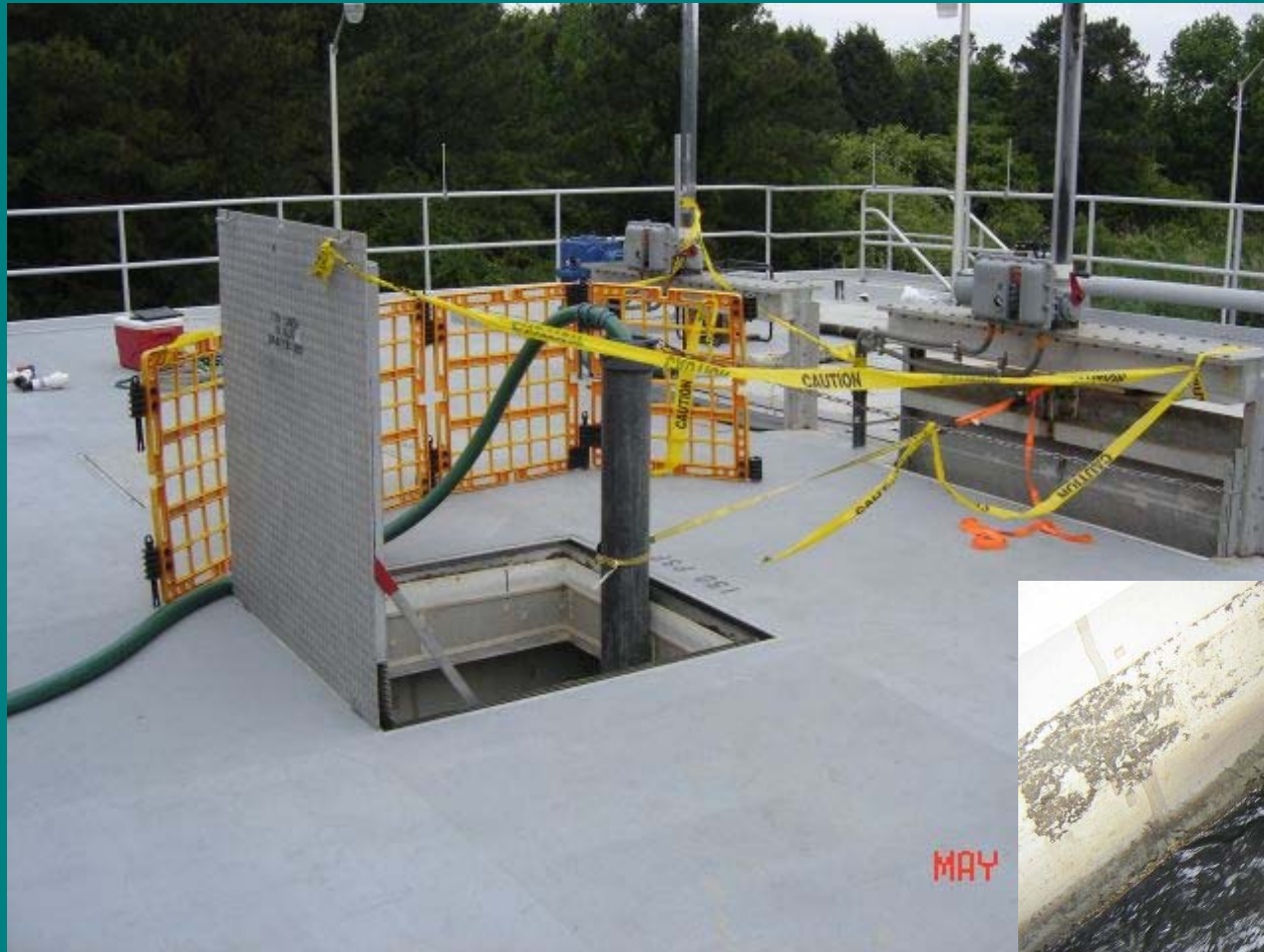
CETP Forced Vortex 24 ft dia Grit Effluent
