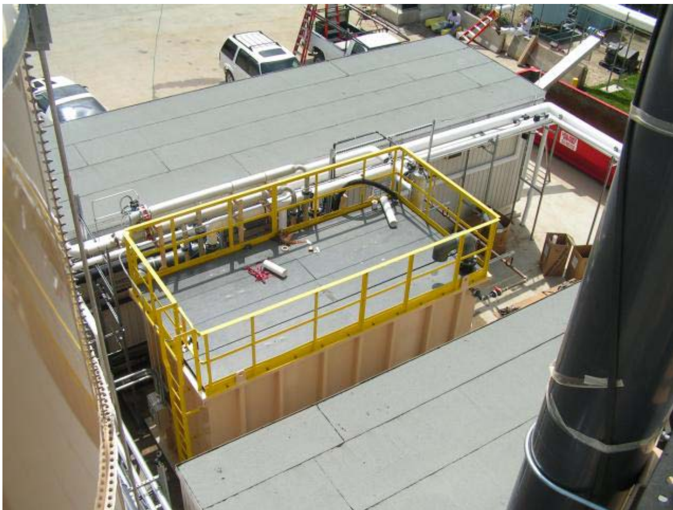
Steel (Above Ground) Membrane Tank
