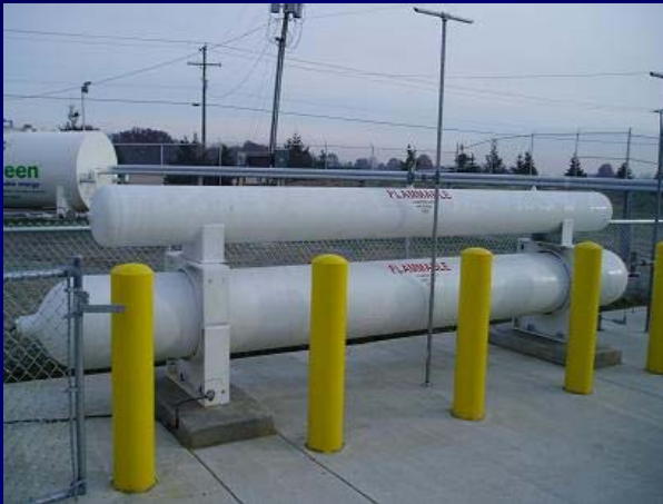
CNG storage tanks
