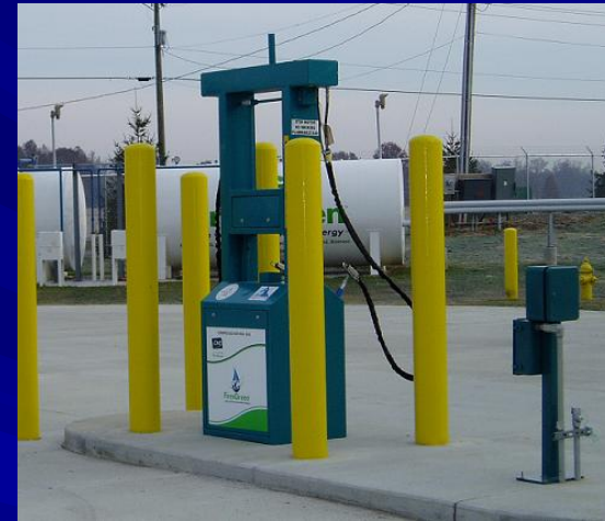
CNG filling station
