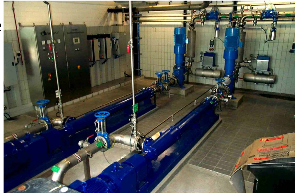
Siemens Crown Disintegrator Wiesbaden WWTP - 60m 3 /hr
